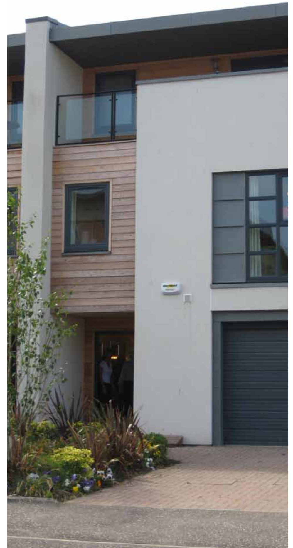
Burnbrae, Edinburgh. Untreated timber within sheltered balcony areas and recessed porch.
