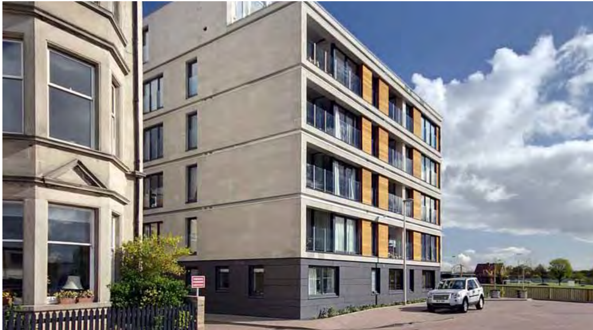
Bangholm Terrace, Edinburgh. Eternit cladding panels at ground floor. Untreated timber at balcony areas.
