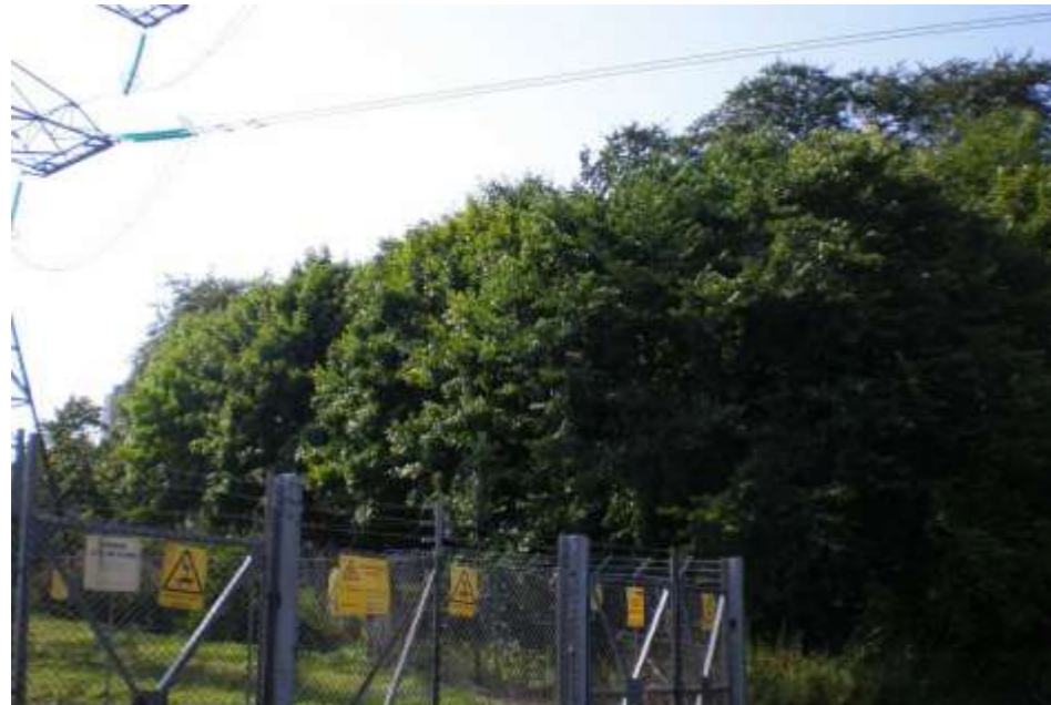
FIG 50: EXISTING SUB STATION COMPOUND
