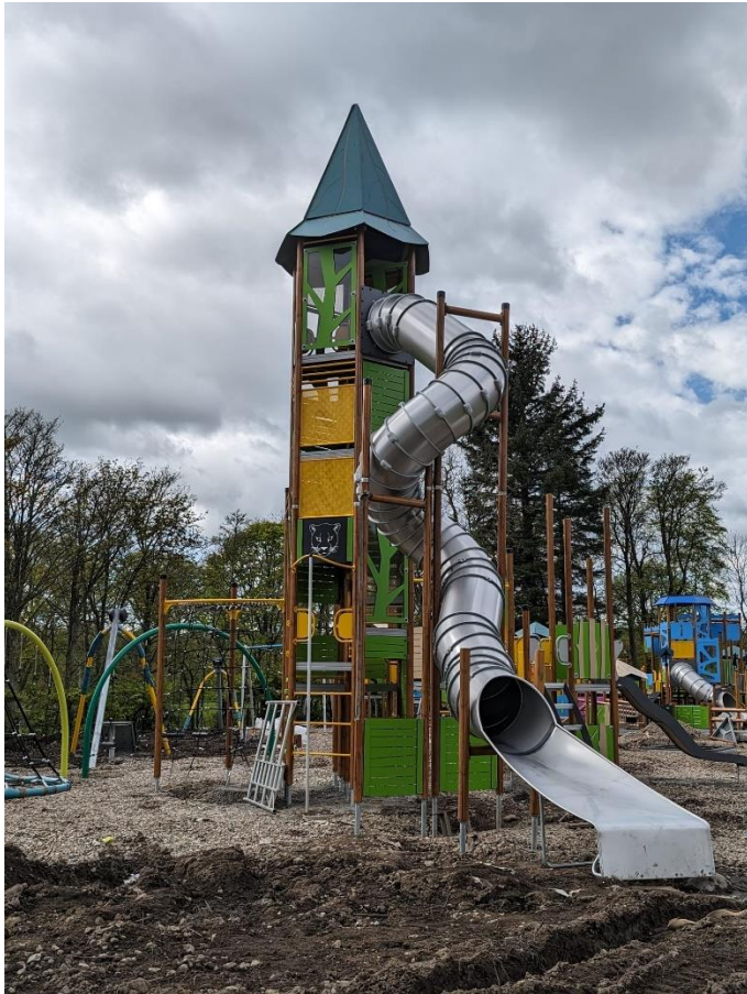
Large tower – more challenging unit with tube slide for older age ranges.
