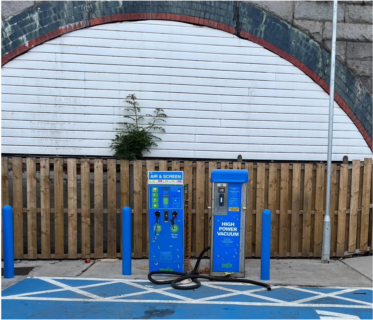
Approved water, air and vacuum units installed at the north of the site.
