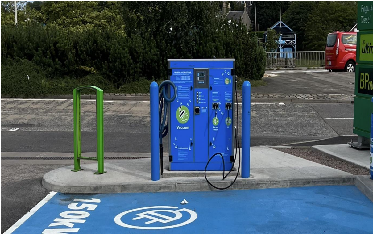
Access to the site is still clearly visible despite the additional water, air and vacuum unit being installed at the entrance.
