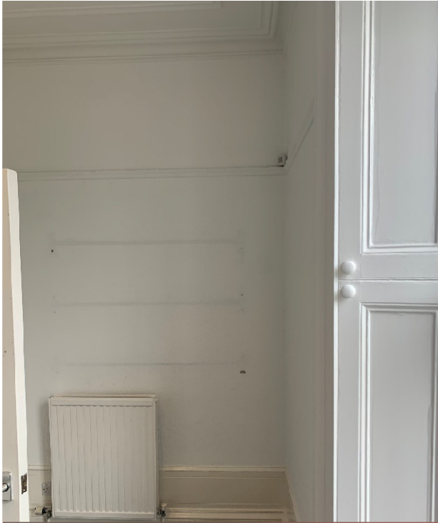
Ground floor skirtings, cornice, picture rail and timber panelling all to be retained
