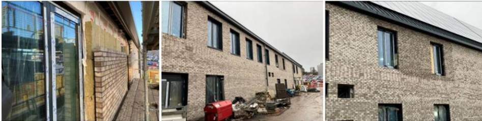
Install of pavers to bereavement suits, backfill fill following lighting protection install works
