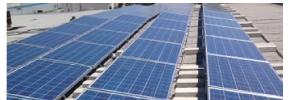
Figure 28: Plot One solar panels
