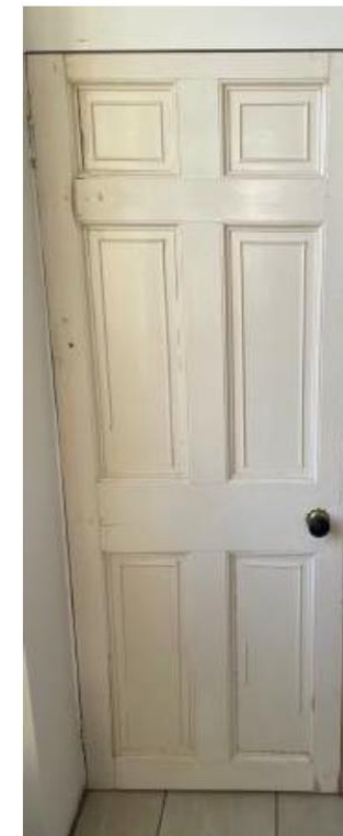
KITCHEN CUPB DOOR
