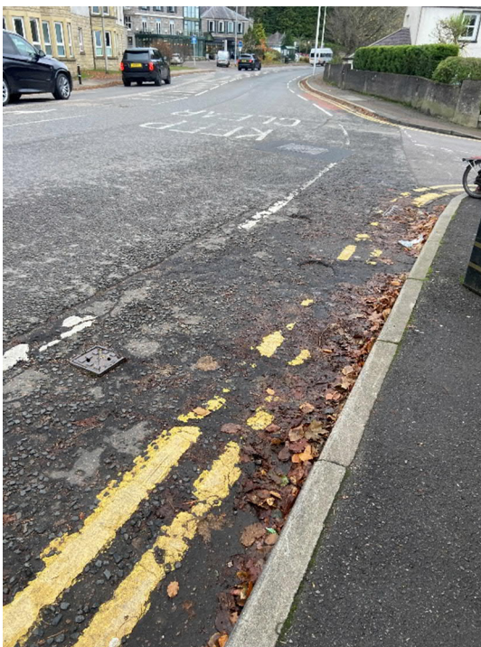
Figure D.2: Advisory Cycle Lane - Poor Surfacing
